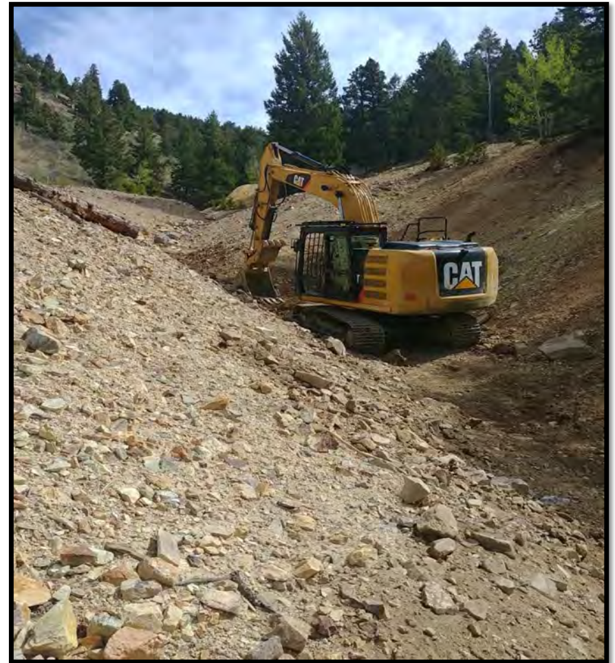
Photo # 3- Preparing Channel for Wall and Riprap. Over 3,000 cubic yards of material had to be excavated in order to expose bedrock. Rebar was drilled into bedrock in order to anchor the wall
