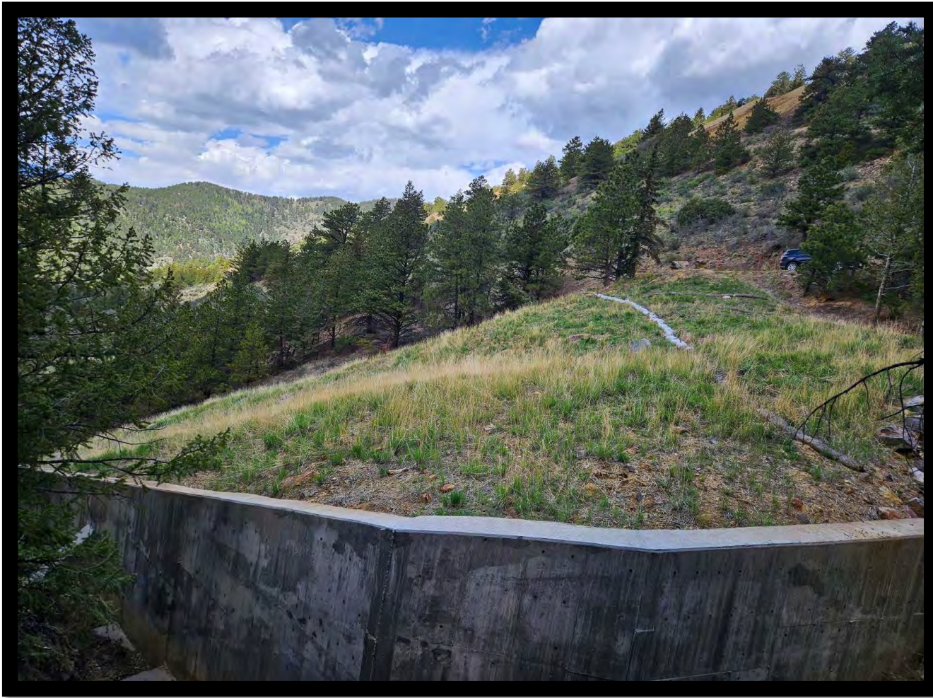
Photo # 8 - Concrete Wall Backfilled with Mine Waste and Revegetated- Over 18,000 Cubic Yards of Material Consolidated Behind Wall
