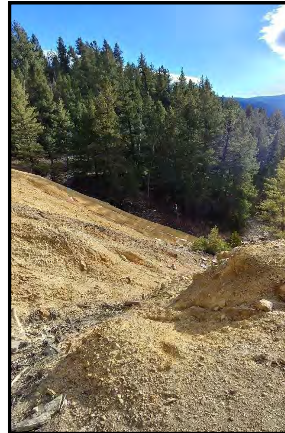
Photo # 2- Casino Mine Pre- Reclamation- Deep Erosion Gullies in Casino Waste Pile with High Concentrations of manganese, cadmium, copper and zinc
