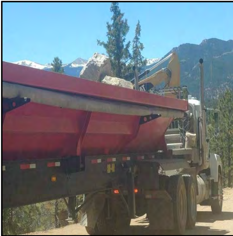
(Left) Photo # 20 Delivery Truck Prior to Dumping Boulders Down the Slope towards Project Manager and Operator
