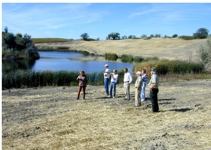
Mark designed and managed this 1999 AML Project at the Custer Mine, near Garrison, ND, that included backfilling a dangerous surface mine highwall and forming a shoreline around an 8-acre trout pond and wetland.
