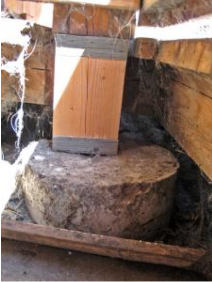
Shoring inserted between foundation and floor joist to keep house level due to subsidence.
