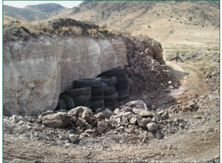
This is believed to be the first use of toroidal tire plugging in a U.S. mine site.
