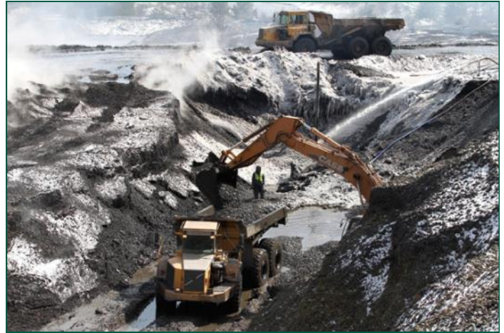
Temperatures fell into the single digits for almost a month while crews worked at Simpson Creek
