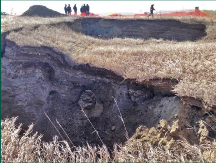
Emergency Sinkhole site meeting with Bowman and Trans Canada officials at the Halleck Mine in 2014.
