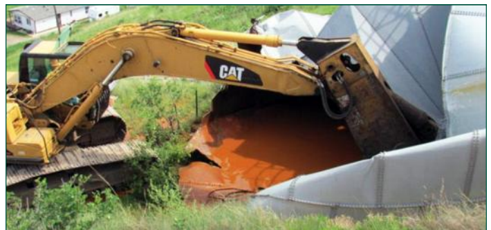
Sludge in existing water tank.
