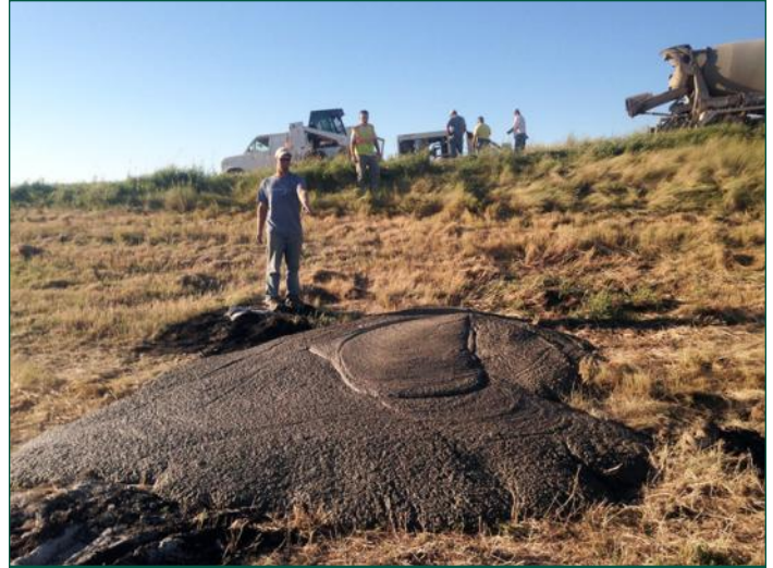
Construction Inspector pointing out the blow out in the south ditch of the east-west road.
