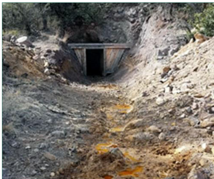
Figure 2: The adit at Lead Queen Mine, pre-remediation. An adit is a horizontal entrance to an underground mine primarily used for de-watering and extraction of minerals during operations.
