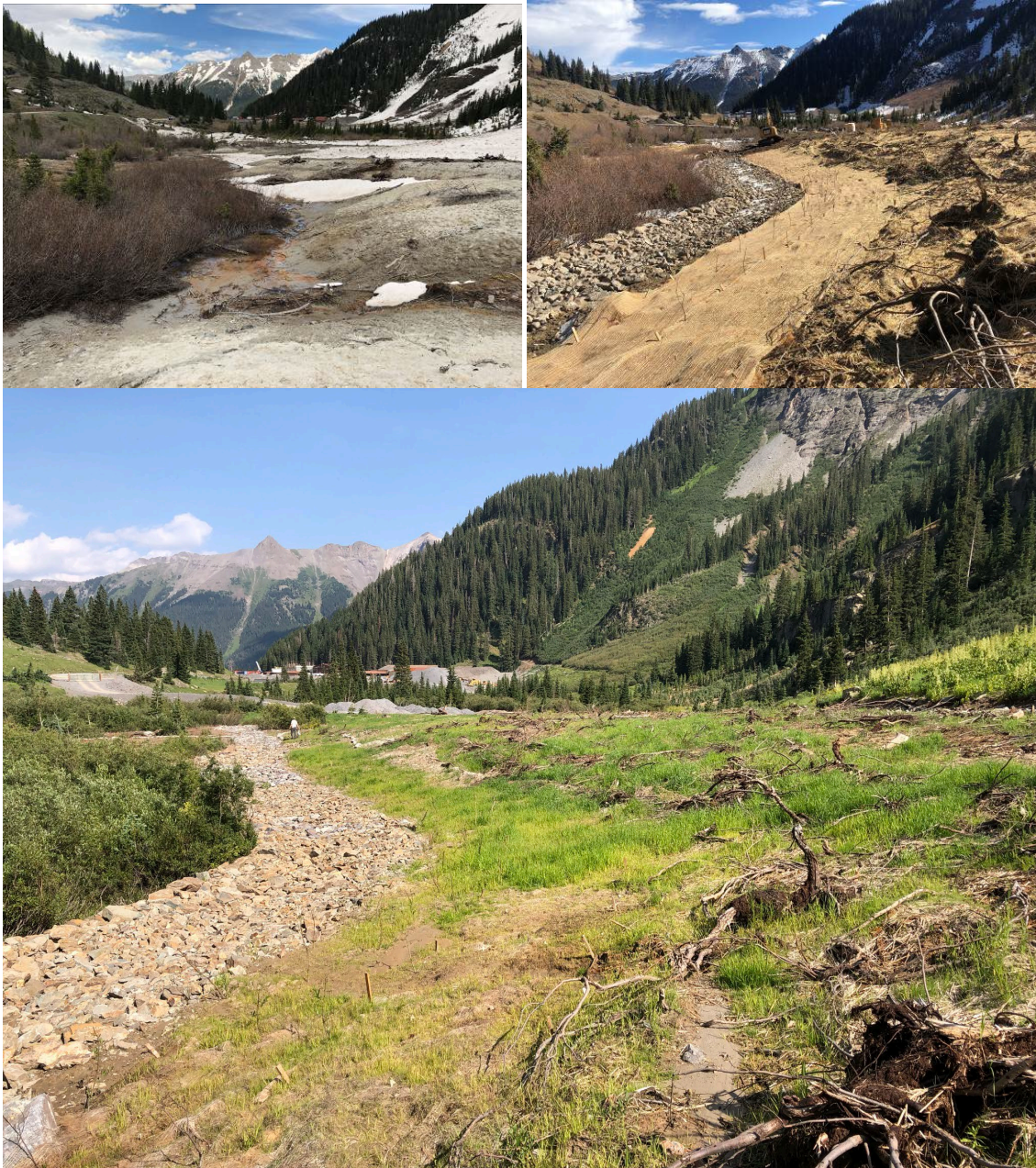
Figure 4: Conditions at grey tailings preconstruction showing toe of slope (left) and after construction (right) showing run-off channel and reclaimed slope, and bottom center 1 year post construction.
