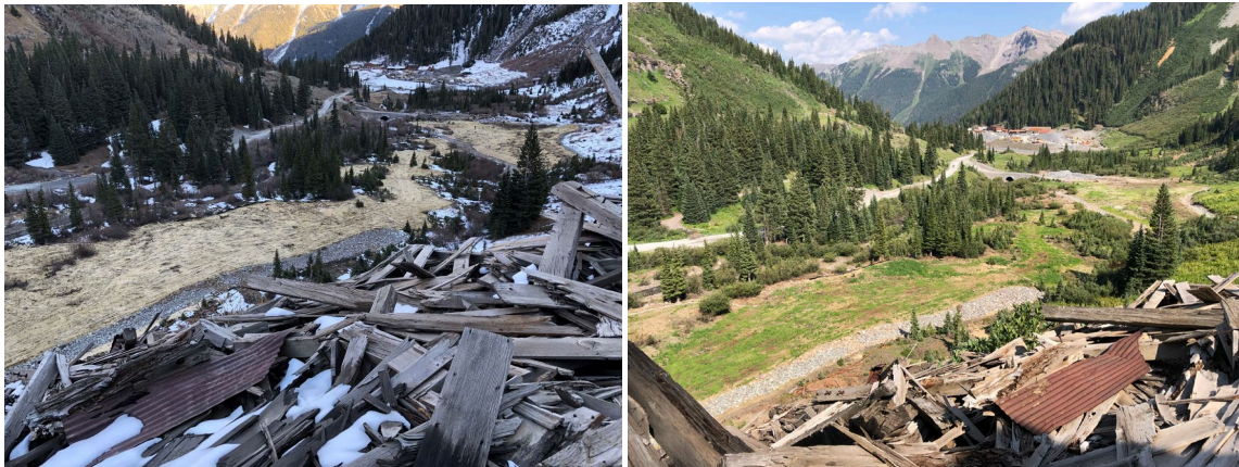
Figure 6: Before conditions (upper left) showing 4.2 acres of yellow and grey barren areas with visible test plots. During construction photo (upper right) showing a partially reclaimed grey area and a graded and consolidated yellow area. After conditions (bottom left) photo showing fully graded, consolidated, and mulched site with constructed drainage controls, and 1-year post construction (bottom right).
